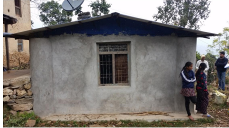
Above: Bottle house under construction. Horizontal and vertical seismic reinforcement bands are for structural safety. Below: Bottle house completed and ready for handover to the earthquake-affected family.
